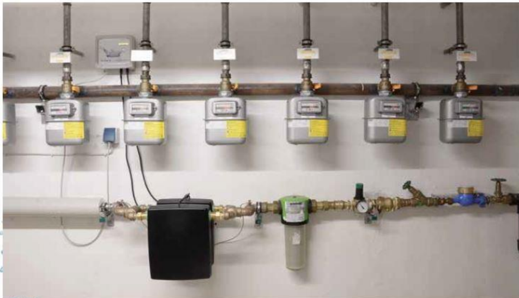
Apartment block with 10 residential units, Würzburg region, Property management: Eichhorn Immobilien GmbH
